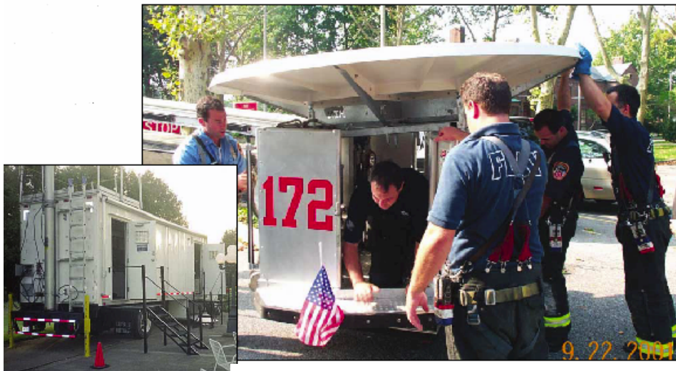
NYSTEC's Deployable Advanced Communications Environment (left). Above, New York's Bravest from FDNY's Ladder Company 172 and Engine Company 330 assist Globecomm in raising a 2.4 meter antenna for installation on top of a four-story hospital.
