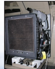
Integrated Diesel Generator
