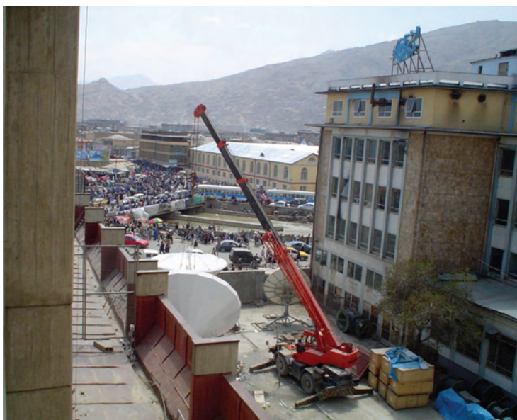
Kabul: Globecomm builds the hub facility and District Communications Network at the Ministry of Communication & Information Technology
