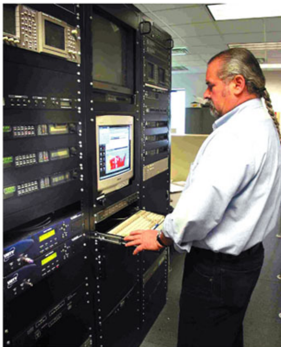
Figure 1. A Globecom technician checks HD-ready MPEG-4 encoders at the IP-PRIME Super Headend.
