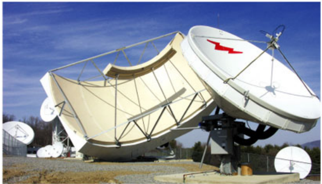
Figure 3. Fixed 7m Simulsat multi-beam antenna and 4.5m motorized antenna provide content acquisition at the SES AMERICOM Super Headend.
